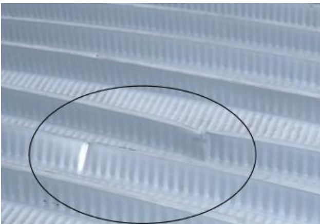
Fig. 4 Local instability before the collapse (Poland)
