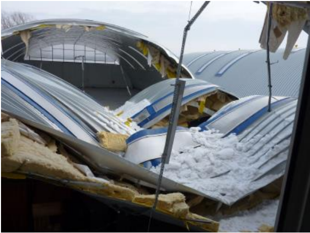
Fig. 3 The ABM building collapse (Poland)
